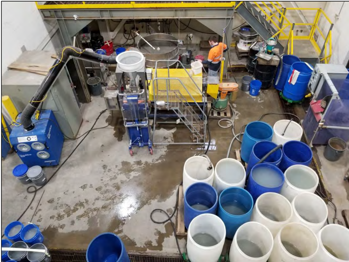
Figure 13-21: Eriez Pilot Plant Ball Mill and Gravity Recovery Circuit
